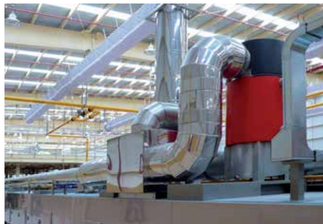
Heat recovery system channels heat from the oven back into the plant
